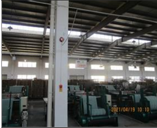
Photo of fire safety equipment Fire alarm.JPG
