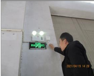
Photo of fire safety equipment Emergency lighting testing.JPG
