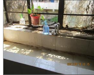
Photo of the sanitary facilities Washbasin.JPG
