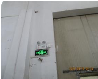
Photo of fire safety equipment EXIT sign and emergency lighting.JPG
