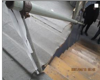
Photo of non-conformity The height of one staircase handrail was not enough.JPG
