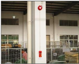
Photo of fire safety equipment Fire alarm.JPG
