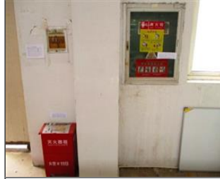
Photo of fire safety equipment Fire extinguishers and hydrant.JPG
