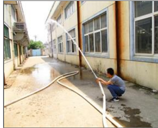
Photo of fire safety equipment Testing hydrant.JPG
